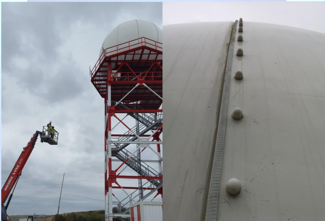
Radar installation and radome structure illustrating physical condition and construction features relevant to performance assessment.
